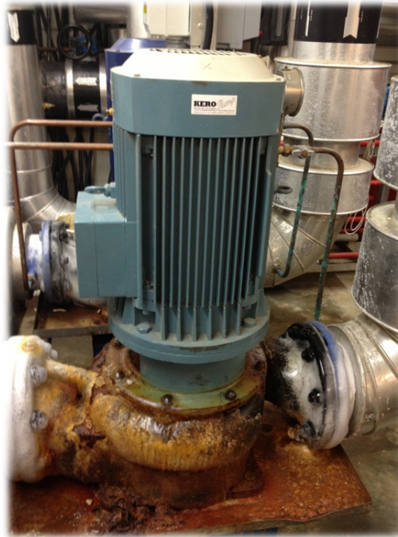
Figure 18: Corrosion phenomena due to a calcium chloride solution
