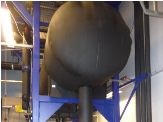
a) CO 2 tank
